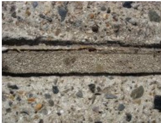
PVC foam still standing proud of concrete since 1969
